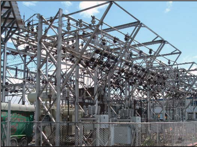
Substation La Uruca
